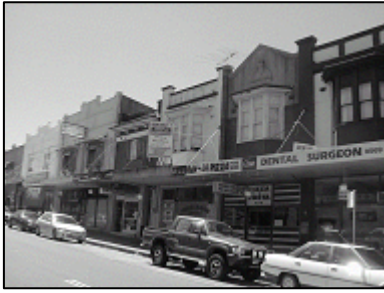
The removal of original window awnings, canopy and bay windows degrades the visual quality of the centre and is to be avoided.
